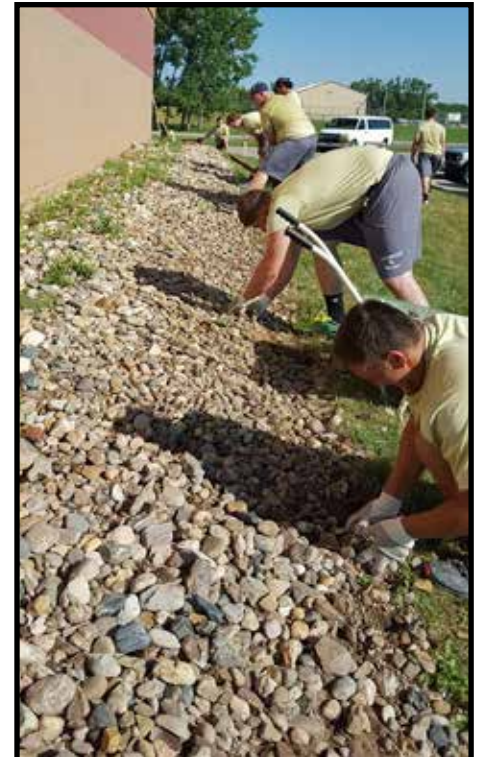
Thank you to members of the Hardrockers football team who worked hard removing rock at Black Hills Works on August 12.
